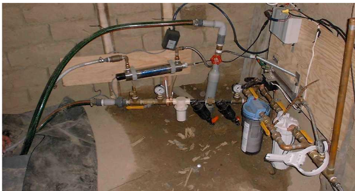
Figure 2. A device for disinfecting water based on ultraviolet lamps is shown.
