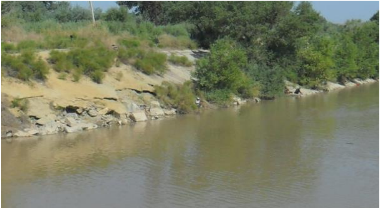
Fig.1. Destruction of the concrete lining of the Anasay main canal
